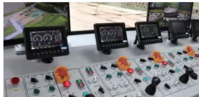
Inside the Centralized Control Room
